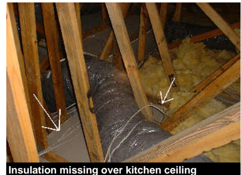
Insulation missing over kitchen ceiling
